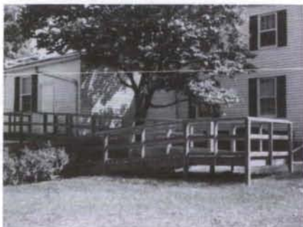
A view of the new ramp from the parking area at the rear of Holt House
