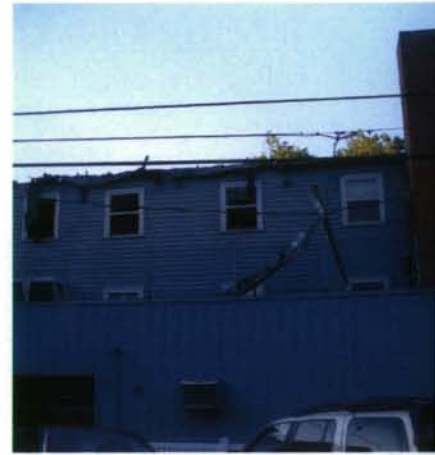
The roof of the Idaho Alpha Chapter house was consumed by the Aug. 1 fire.
